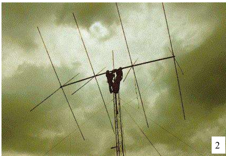
A 4-element amateur radio quad antenna. The two men working on it show the scale. The wire loops are almost invisible, suspended on the ends of the crossed supports
